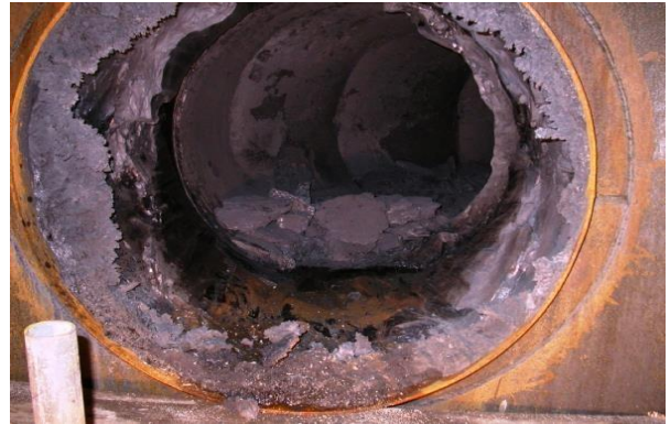
Fig -1: Fouling in chimney
